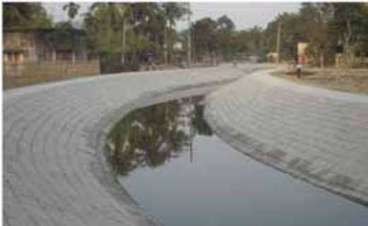
Urban drainage channel
