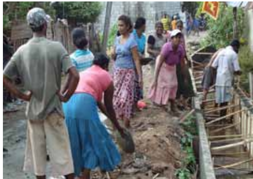
Drainage and road improvement done by a community-based organization under Community Contract System in Moratuwa
